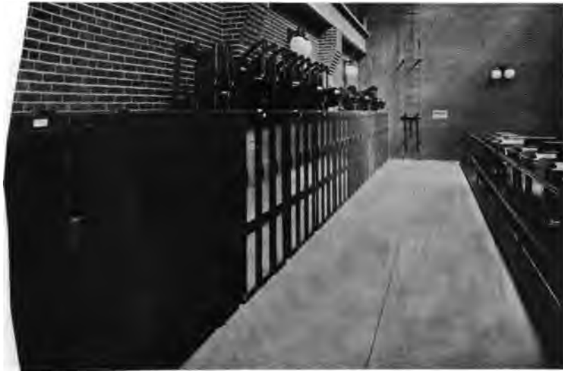
Fig. 3. High-Tension Station. (Boston Elevated Railway Company.)
